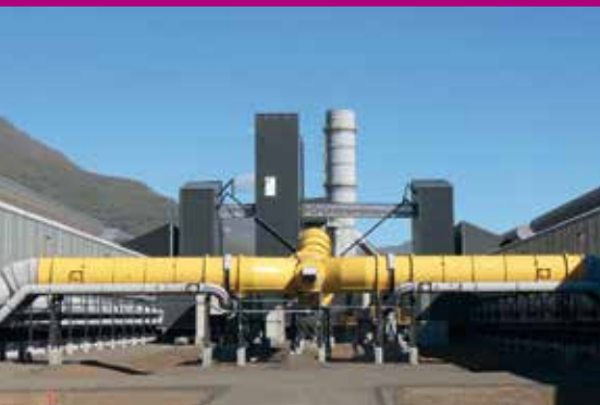
Gas Treatment Center - Alcoa Fjarðal (Iceland)
